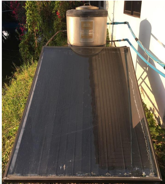
Figure 22 Solar collector system.
