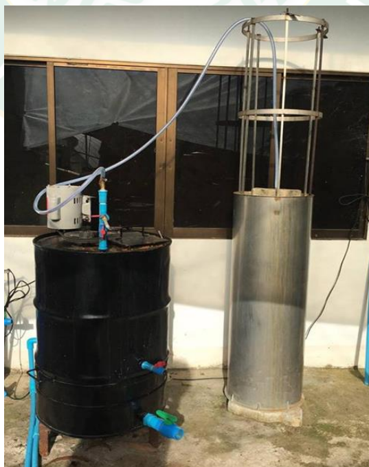
Figure 20 200 L biogas digester system.
