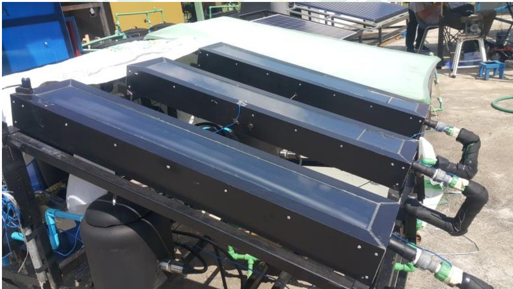
Figure 20 The novel and conventional solar collector (PCM1,PCM2 and without PCM) installed.
