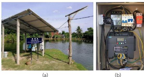
Figure 3 Aquaculture ponds (a) Solar panel in aquaculture ponds (b) Solar Hybrid Inverter in aquaculture ponds
